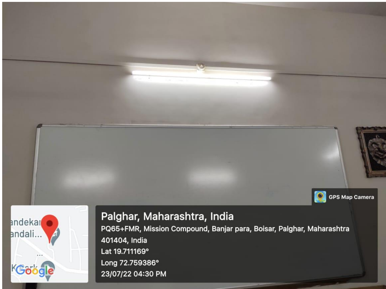
Energy Saving LED Lights in Classrooms
