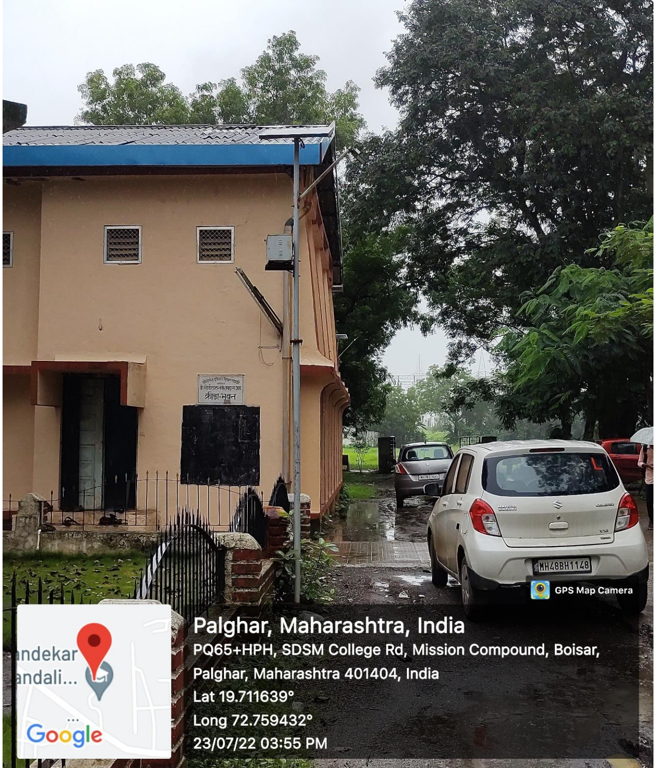
Solar Street Lights in Campus
