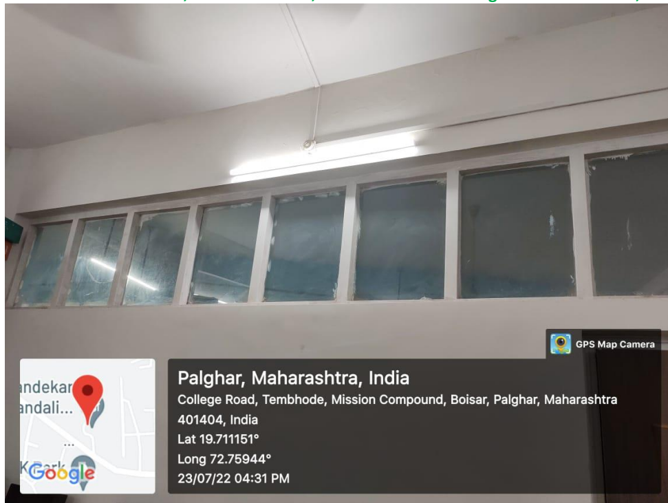
Energy Saving LED Lights in Classrooms
