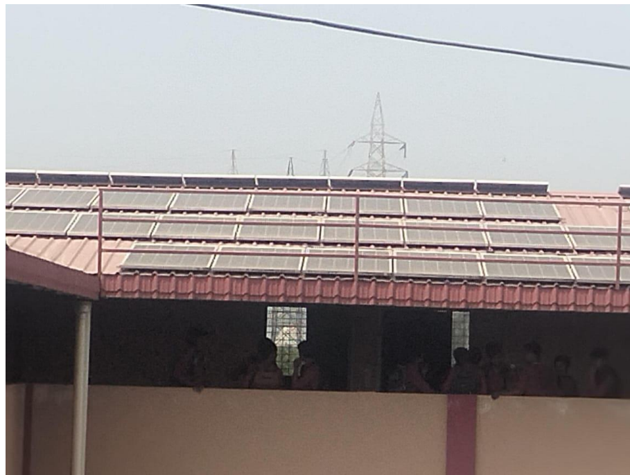
SOLAR PANEL ON THE ROOF
